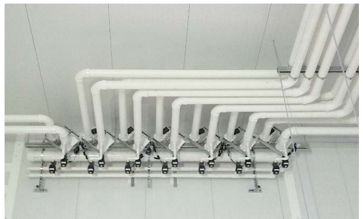
Series IV CA Piping Manifold in Hallway
